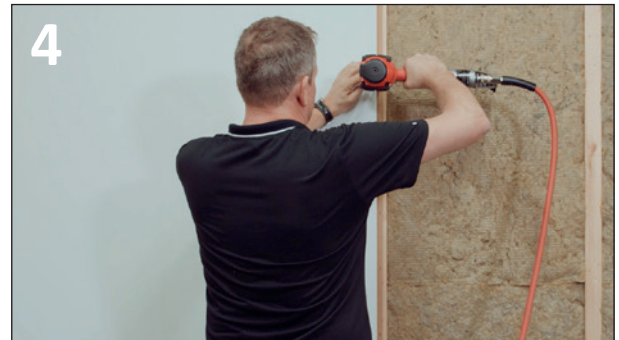
FIT LEFT TO RIGHT FROM A CORNER, OR FROM RIGHT SIDE OF A DOOR OPENING.
